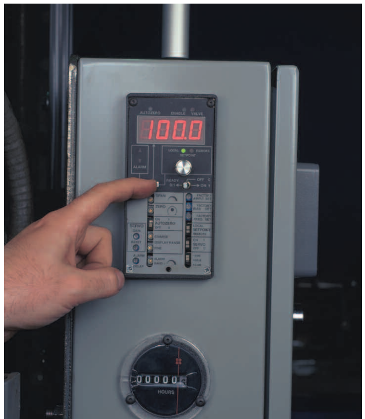
Figure 16. Original factory 100 amp setting
